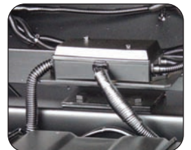
Water Tight Electrical Junction Box and Wiring Harness
